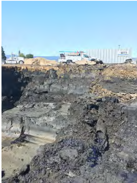
Photograph 3 (13 June 2019): Discovery of section of pipe with semi-solid petroleum product.
