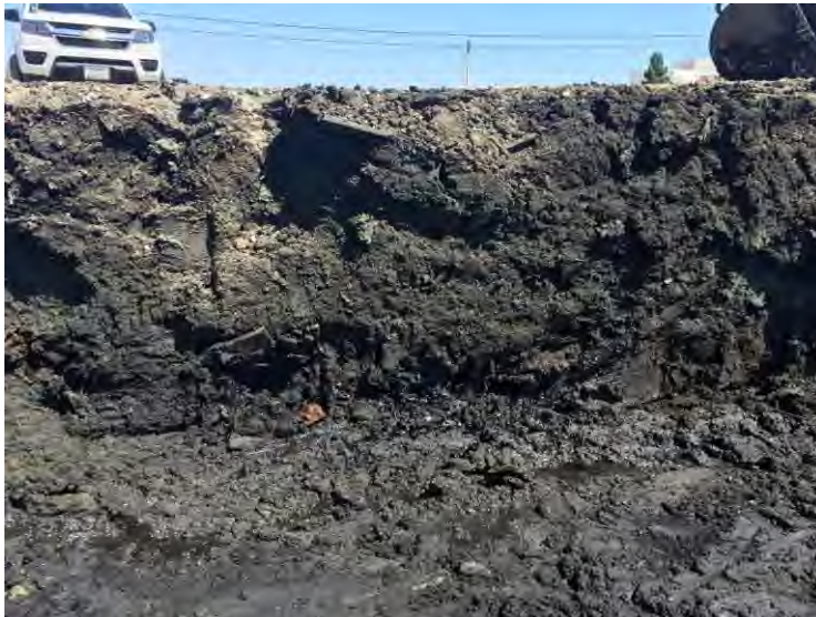
Photograph 1 (12 June 2019): Initial discovery of unexpected heavily degraded petroleum hydrocarbons in Excavation Area E. Photograph looking at southeast wall of Excavation Area E.
