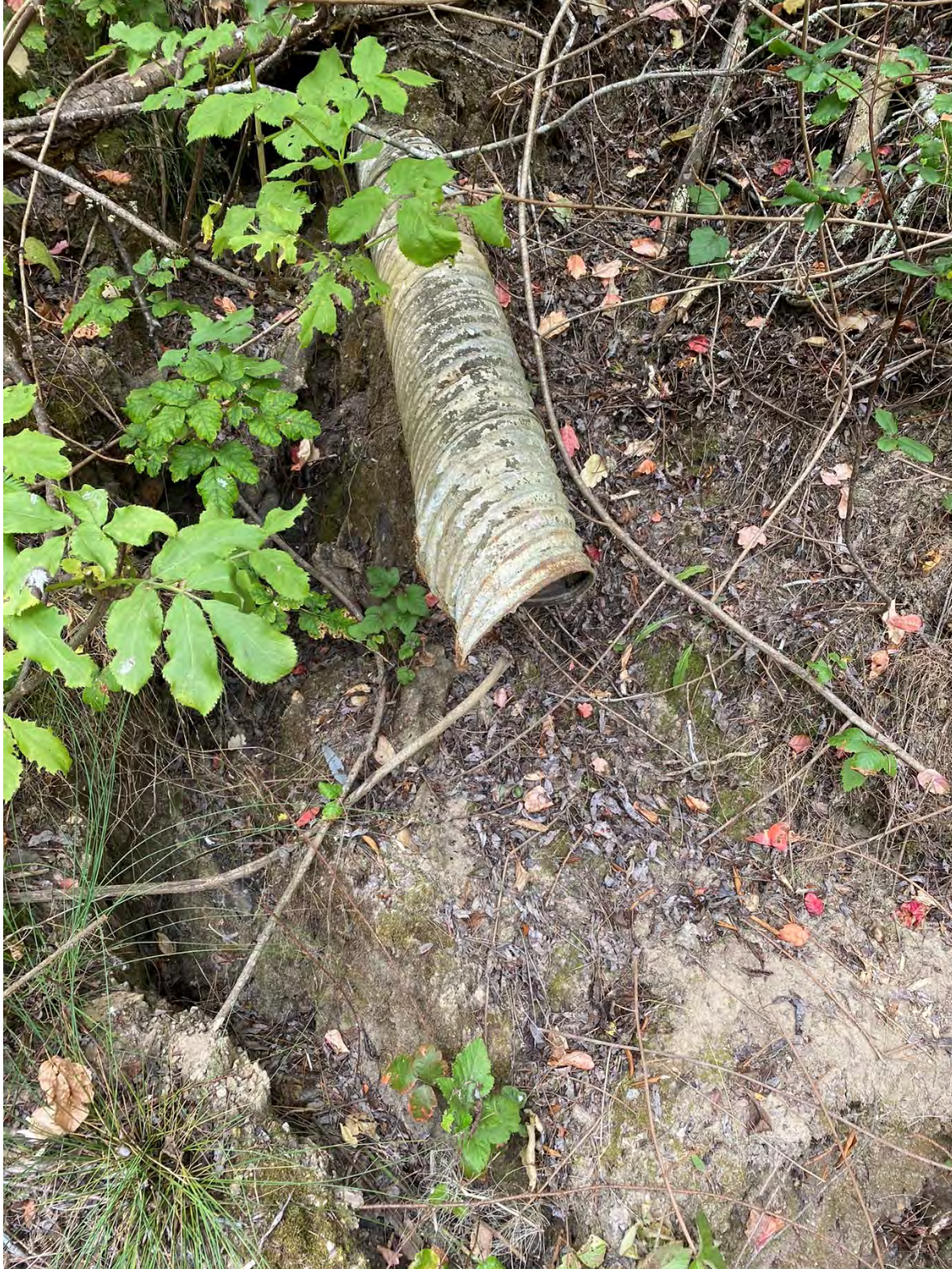
Photograph 2: Ano Nuevo SP, SR-1, Facing west from east side SR-1 embankment; shows disconnected CSP down drain #2 [07/22/2020]
