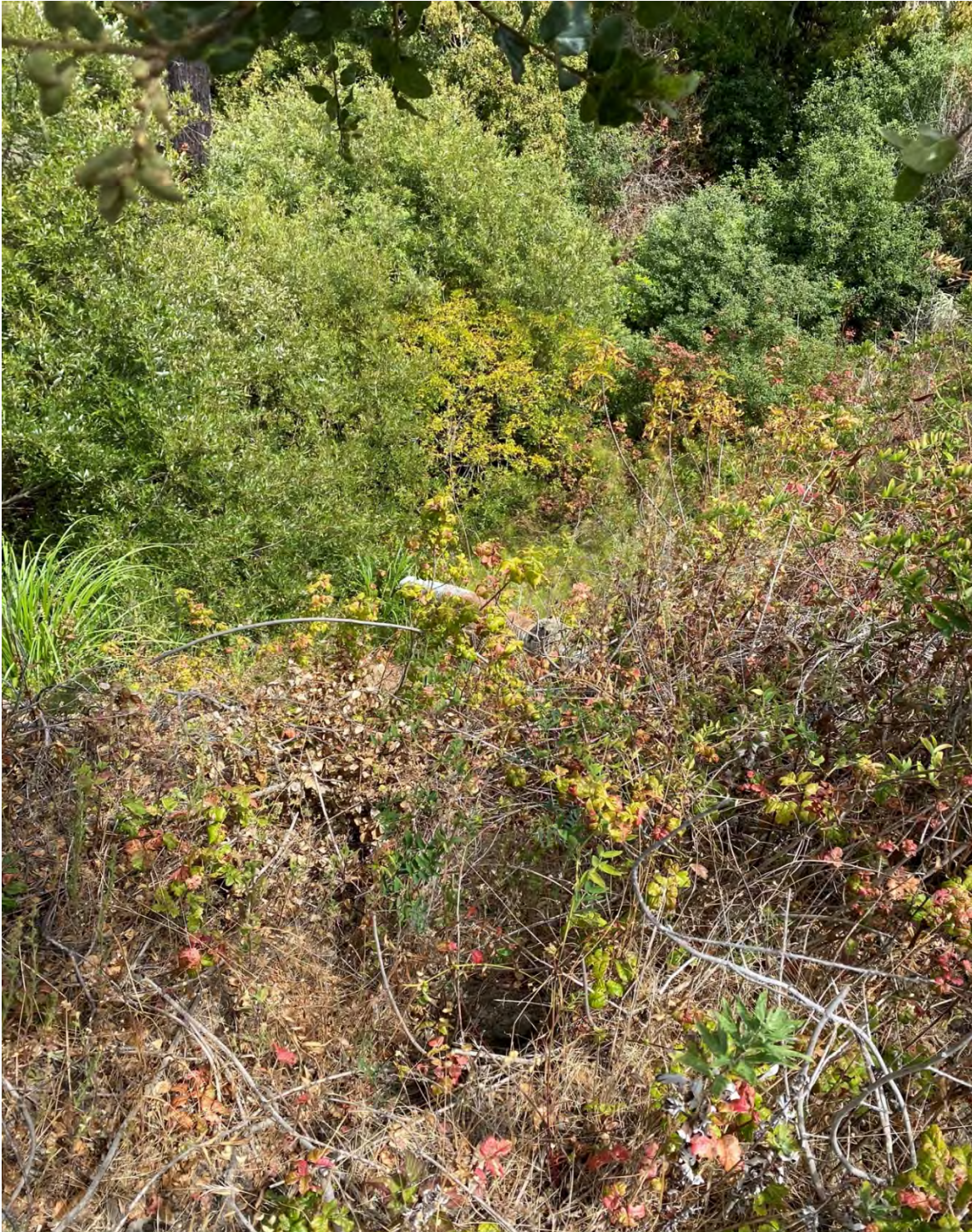
Photograph 8: Ano Nuevo SP, SR-1, facing east from NB shoulder of SR-1; shows CSP down drain #1 to be removed during construction [07/29/2020]
