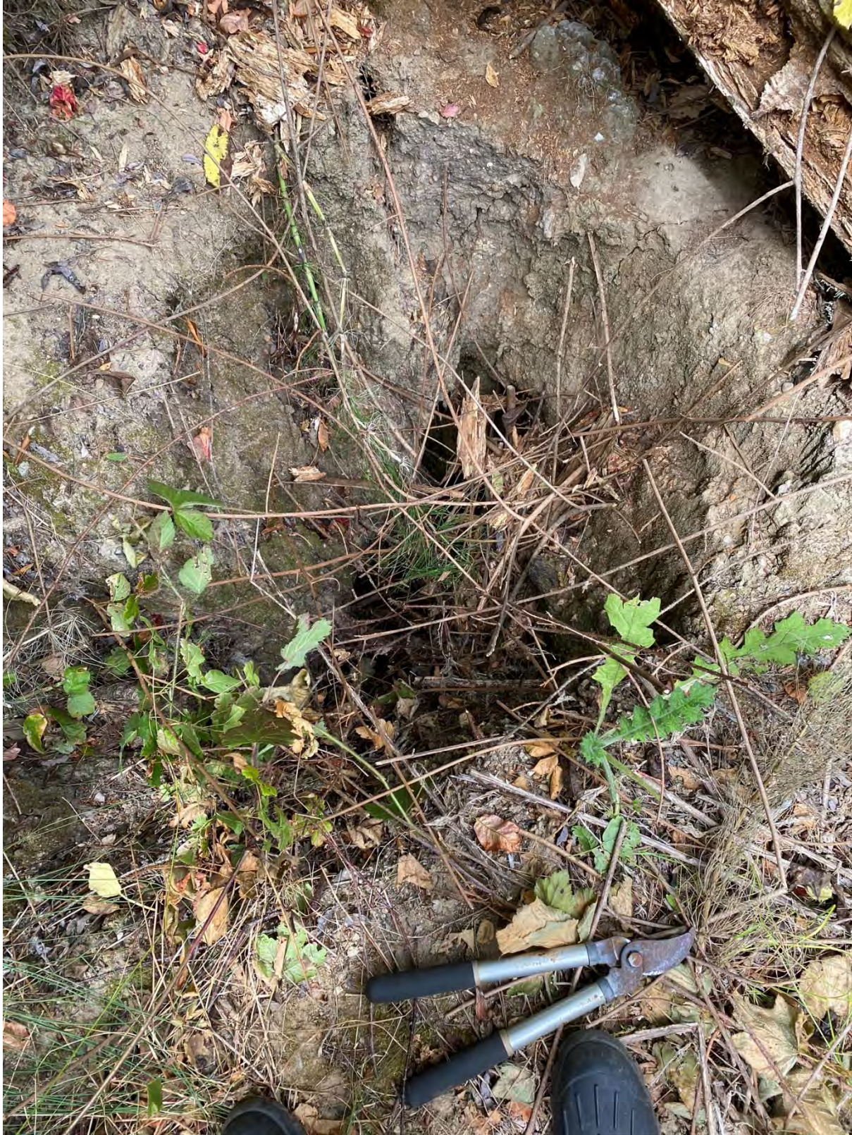
Photograph 3: Ano Nuevo SP, SR-1, facing west from the east side of SR-1 embankment; shows gully created by decommissioned CSP down drain #2 [07/22/2020]
